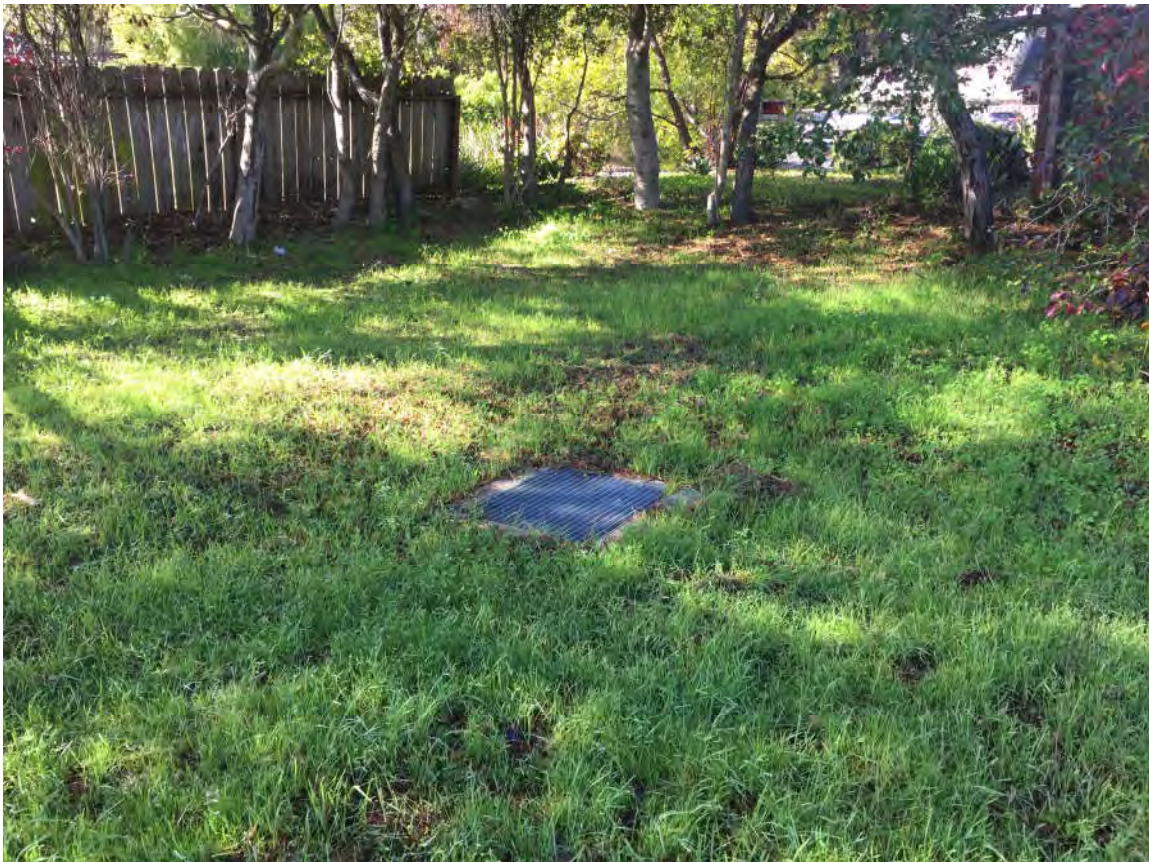
STORM DRAIN LOCATED ALONG WESTERN BORDER OF 1412 CAPITOLA ROAD
